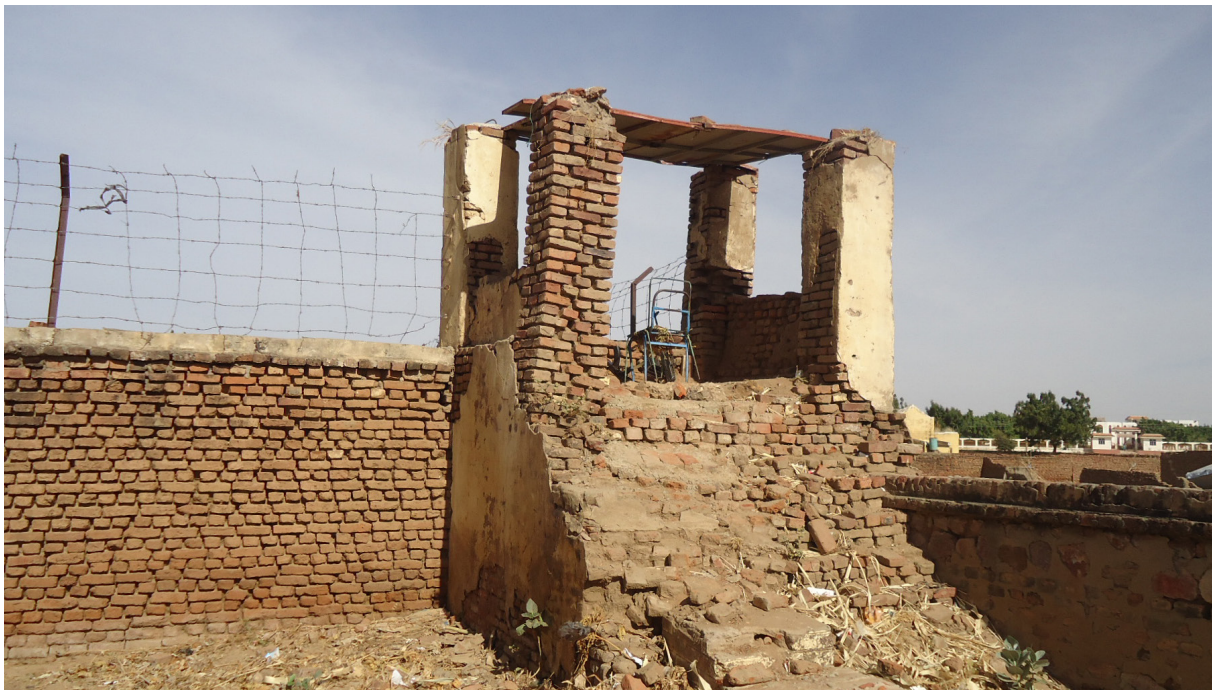
Figure 3: The picture above shows Armata Prison's dilapidated infrastructure.
