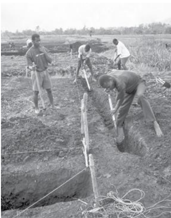
Plate 3-2: Pegged out fish pond and core trench digging. The core will be packed with soil containing not less than 30% clay before dyke construction begins (Source: Ngugi et al.2007).
