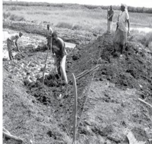
Plate 3-1: Pond construction typically involves excavating the inner area and using that soil to build the embankments (Source: Ngugi et al.2007)
