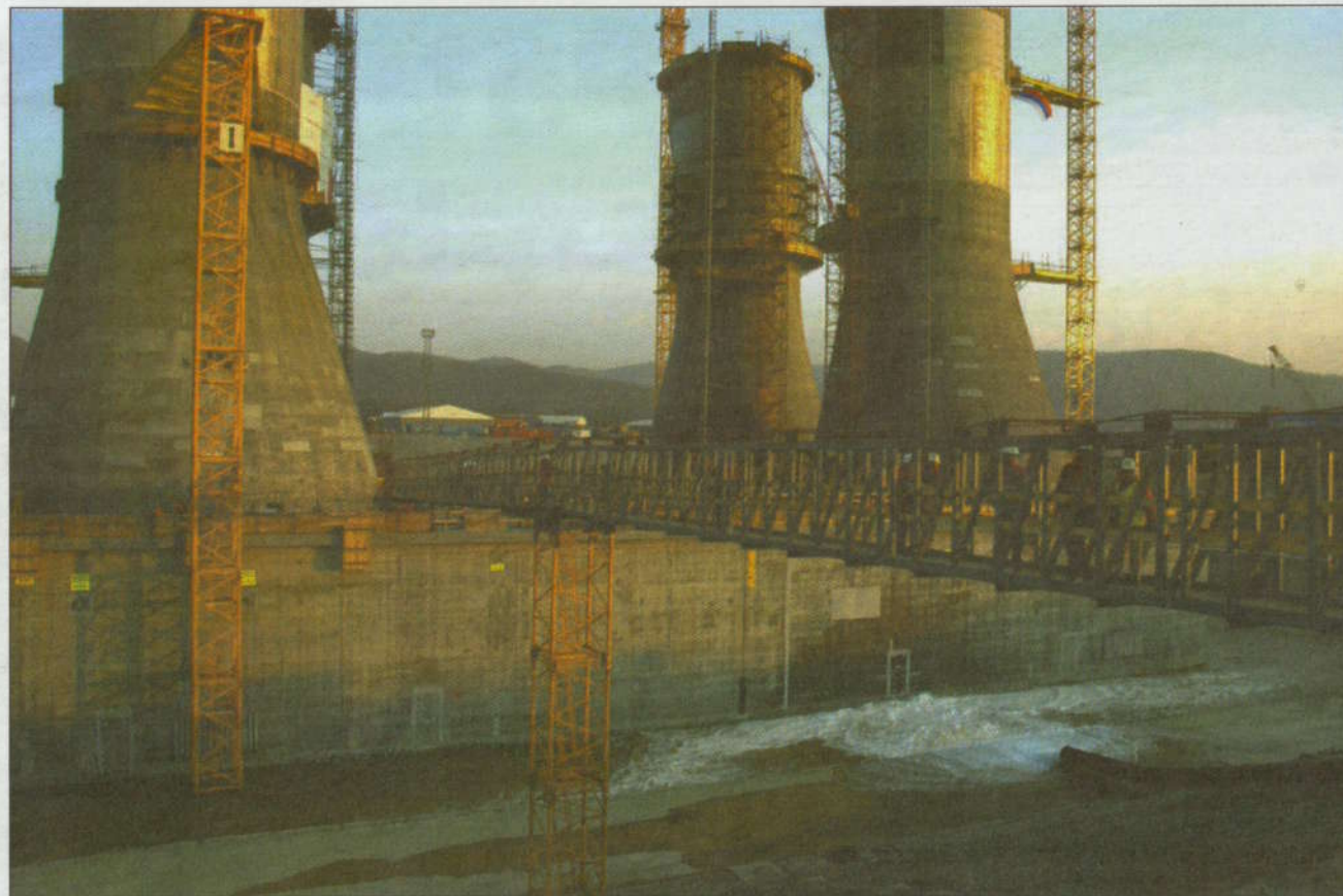
COMPLEX MATTERS: The two concrete gravity base structures of the Sakhalin-2, a long-term oil and gas exploration project, are now complete and weigh a combined 210,000 tonnes.
